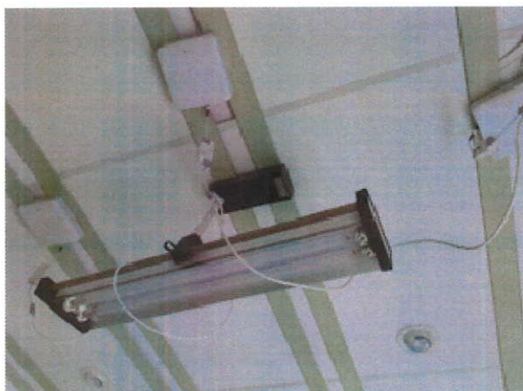
Photo 1. The tested lamp set, installed on the ceiling, used to assess the reduction of microbiological air contamination
