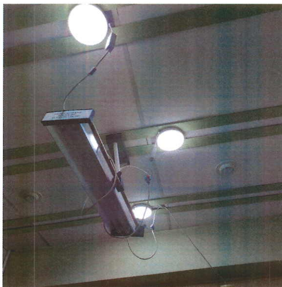
Photo 1. The tested lamp set, installed on the ceiling, used to assess the reduction of microbiological air contamination
